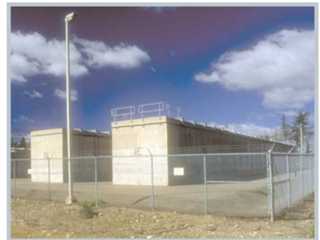
Solid low-level radioactive waste storage, Point Lepreau Generating Station, New Brunswick
